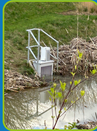
Figure 1 & 2. (Right) Portable gauging station installed by RDN
