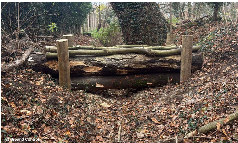
Example of a leaky barrier
